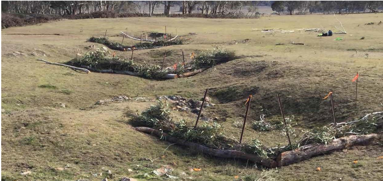
Figure 19. Freshly constructed log and brush weirs temporarily detain flow and collect sediment and nutrients through a steeper section of the valley floor.
