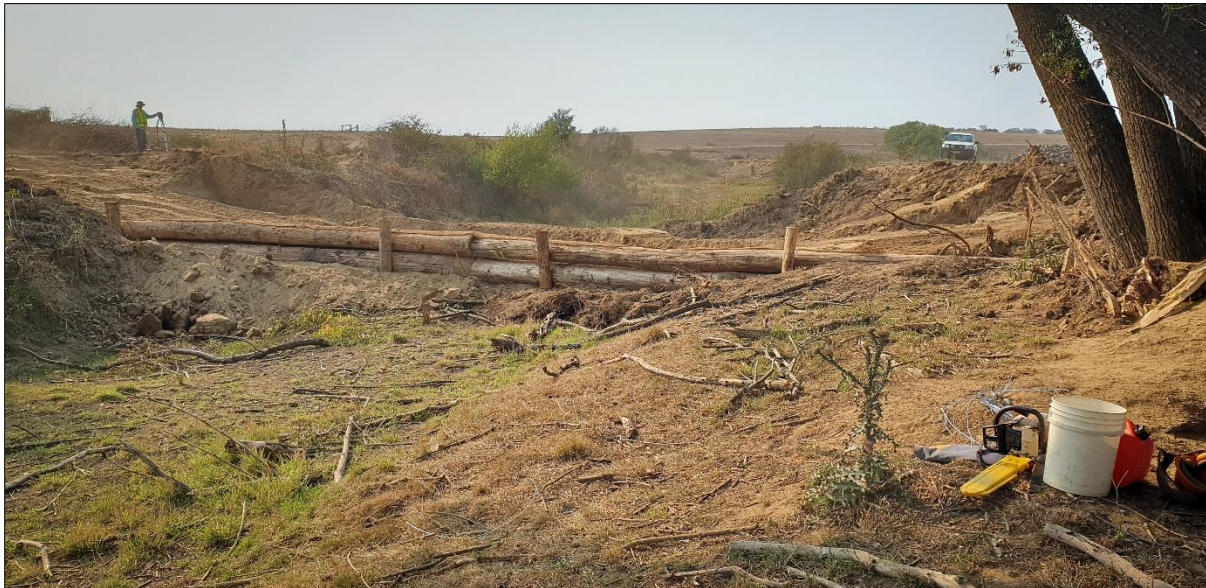
Figure 21. Leaky weir and crossing under construction on Mulloon Creek at “Duralla”, February 2020.
