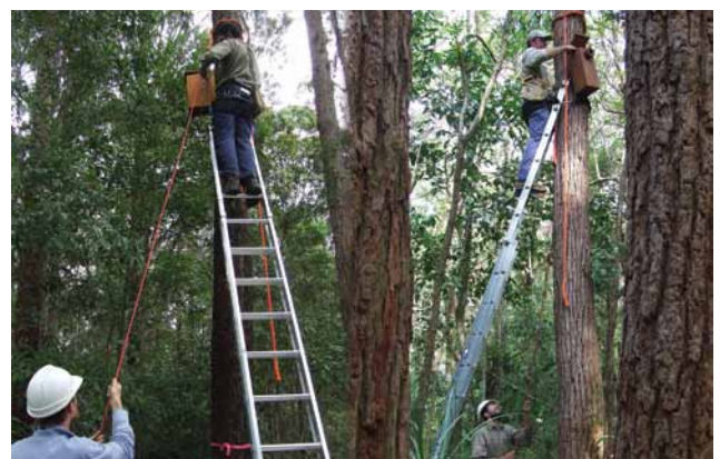
Nest boxes being installed using a sling and pulley system. Person on the ground can raise the box into position and hold it in place until it can be securely attached to the tree.
